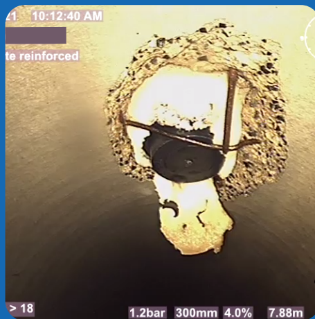
Defect identified for repair
